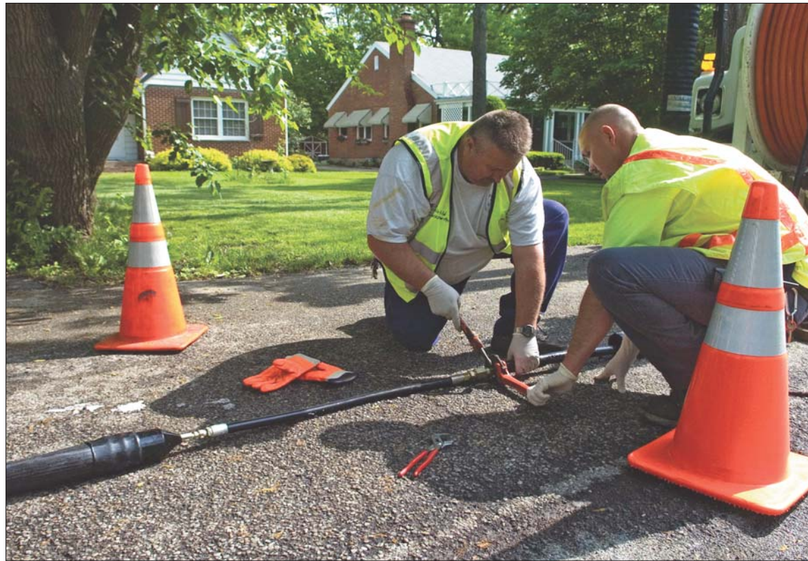
Maintenance operator Kim Campbell, left, and collections laborer Chris Croucher disassemble equipment after applying a root treatment.
