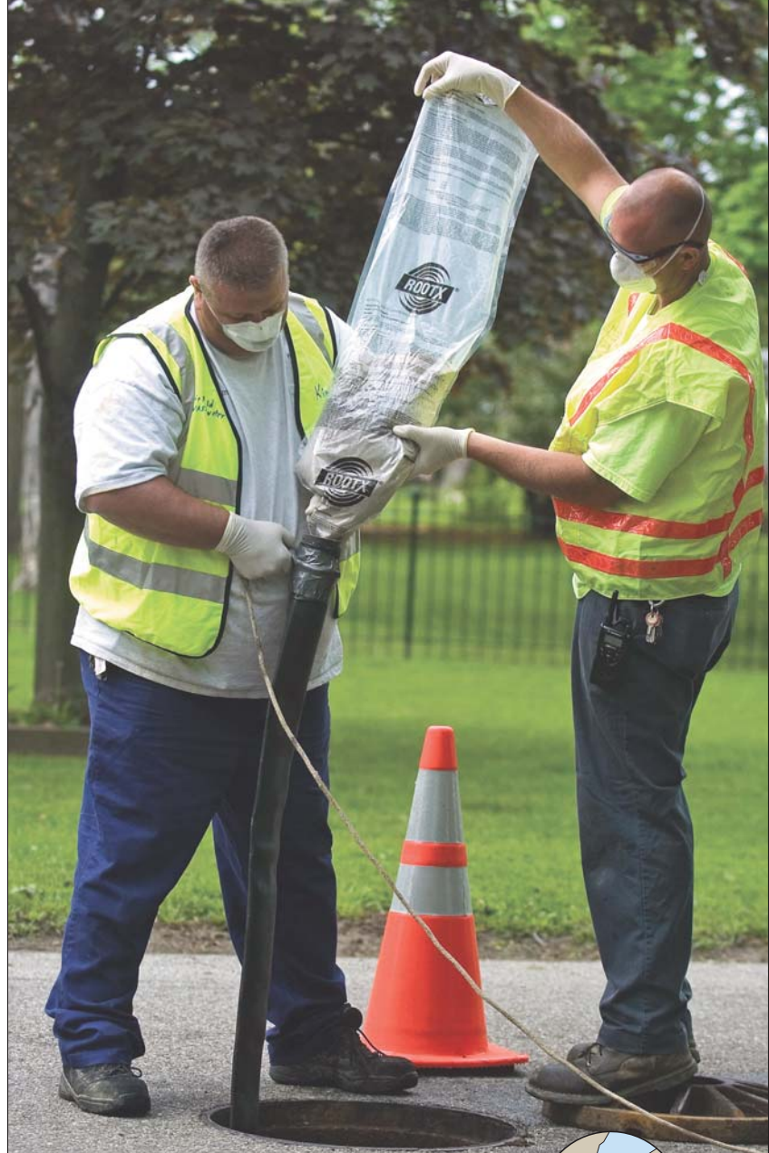
City of Fairfield maintenance operator Kim Campbell, left, and collections laborer Chris Croucher add RootX root treatment to a sewer line. The material, which foams on contact with water, is designed to kill roots in municipal and residential lines. (Photography by Carrie Cochran)
