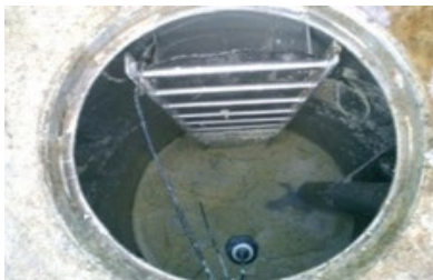
Grease build-up in wet well before
